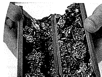
Pipe clogged with zebra mussels
